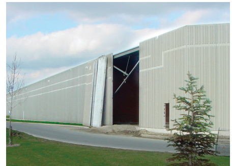
Installation of relocated and new panels to complete the exterior of the expanded area.
